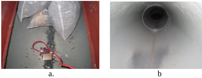
Fig.5. ZigBee communication testing in T-NWK stainless shiny horizontal pipe. a) Pipe full of garbage. b) Pipe without garbage.
