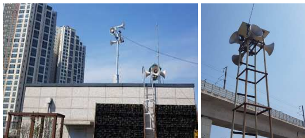
Figure 6. The Automatic voice notification system(left) and village broadcasting system(right) at Cheongju-si plays voice earthquake information
