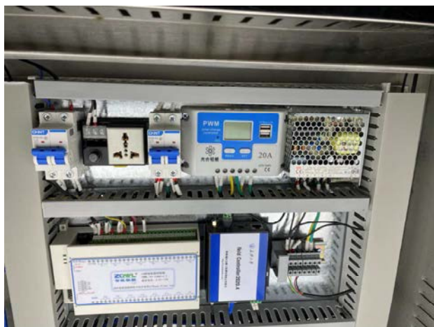
Figure 5. On-site monitoring station
